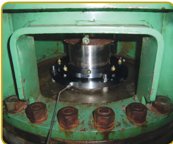
MECO SEAL ON TOP ENTRY REACTOR AGITATOR
